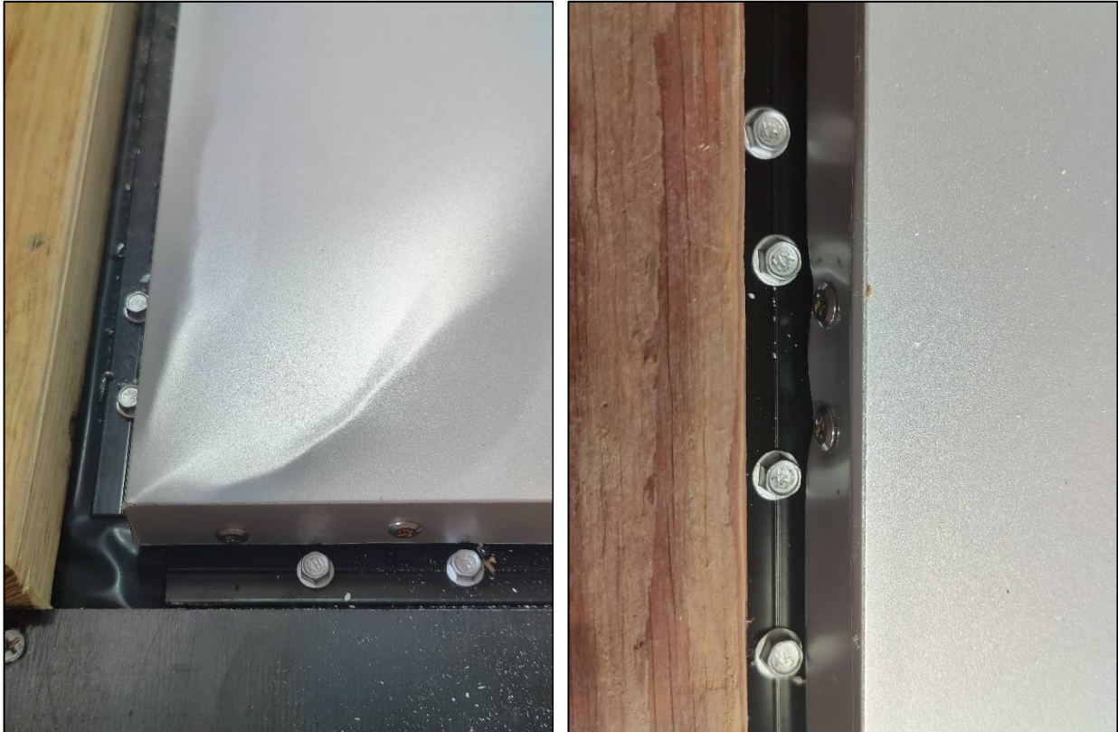
Figure 8: Typical deformation to panel skin in corner (left) and along edges (right)
